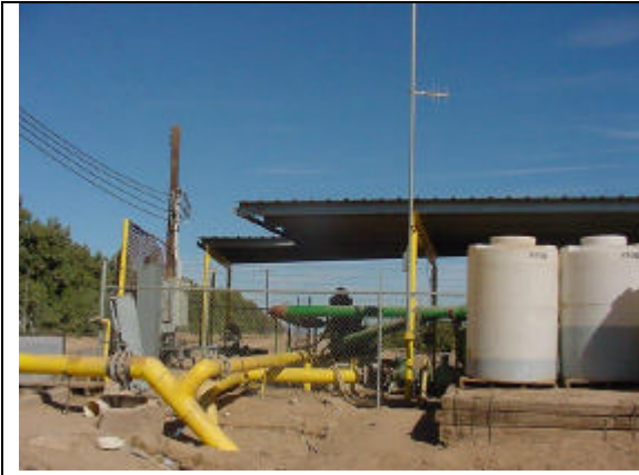
Pump back to canal and direct into filters
