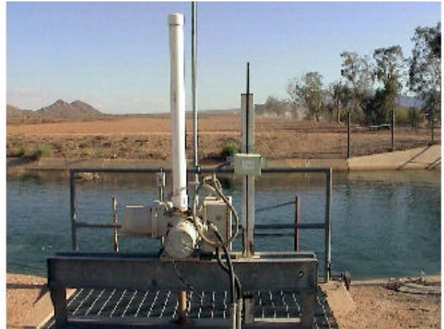
Canal Automation System Located at the Maricopa Stanfield Irrigation and Drainage District. Approximately 87,000 Acres
